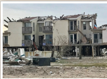
Mexico Beach Florida after Hurricane Michael. Photo: Gladys Cook, Florida Housing Coalition
