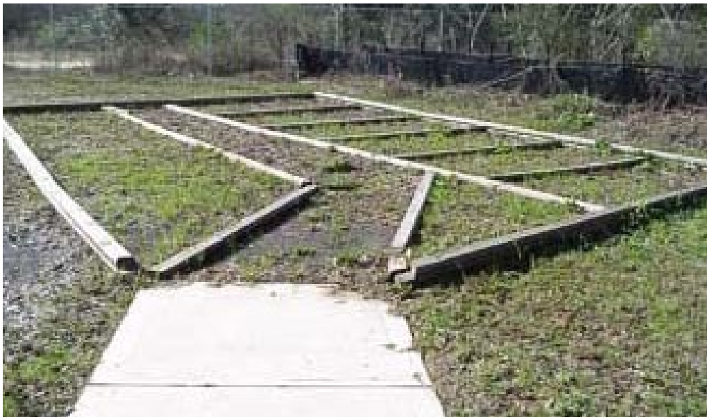
Not Acceptable No fence; overgrown with weeds.
