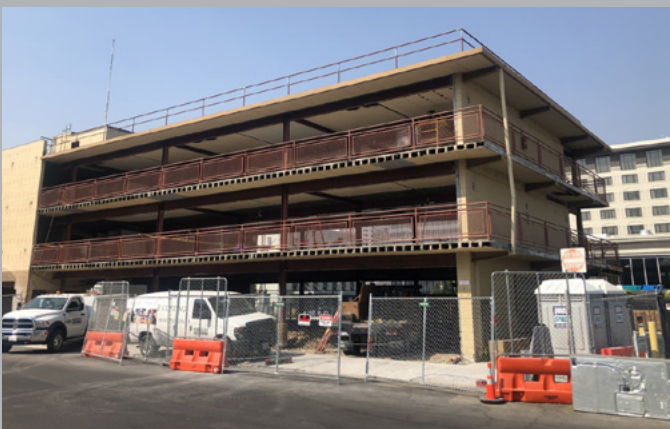
Construction shot showing the shell of the conversion of an old motel to housing for people experiencing chronic homelessness Reno, Nevada
