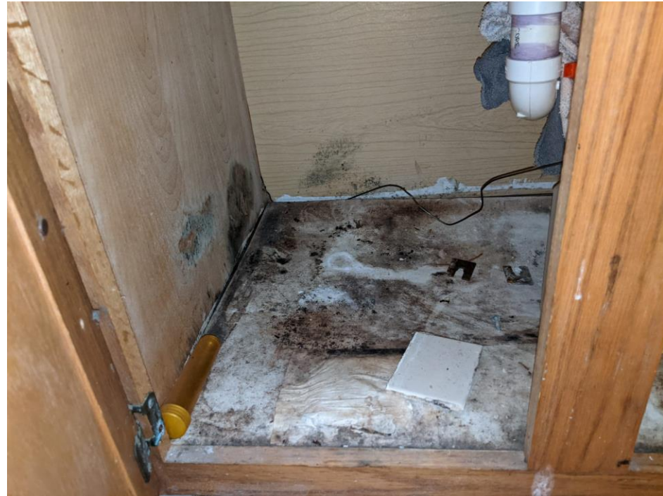
Picture taken 6/6/2021 - tenant has been waiting on sink repair since 2019
